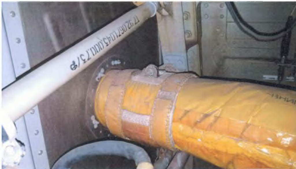
Figure 13. Air bleed duct.
