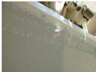
Figure 3-4: Example of ice accumulation along the edge of the lower part of cargo door
